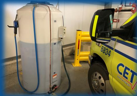
CT04 Outside/Indside tank
